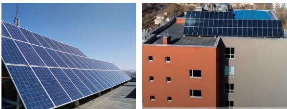
Figure 3. 15 kW solar power system installed on the roof of the MUST
