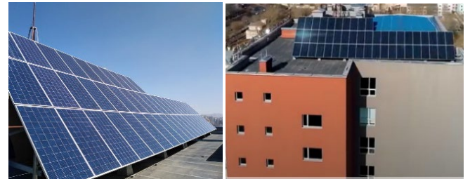
Figure 4. 15kW solar electric system installed on the roof of the 8th building of the Mongolian University of Science and Technology
